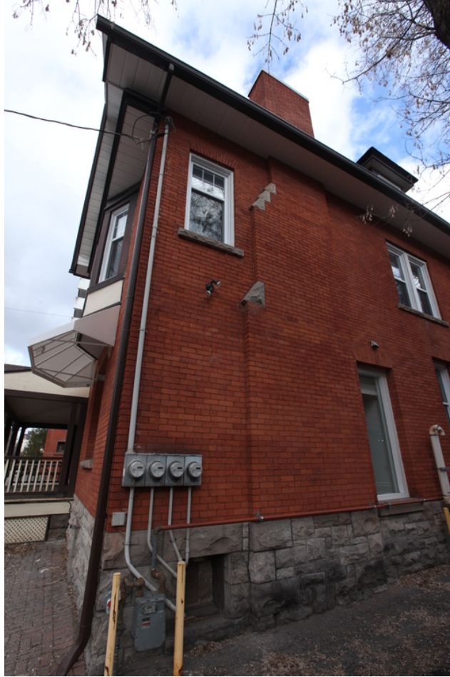
West side of house showing emergency door added in 1963. The door was converted to a window in 1983, and the porch demolished to improve access to the parking lot.
